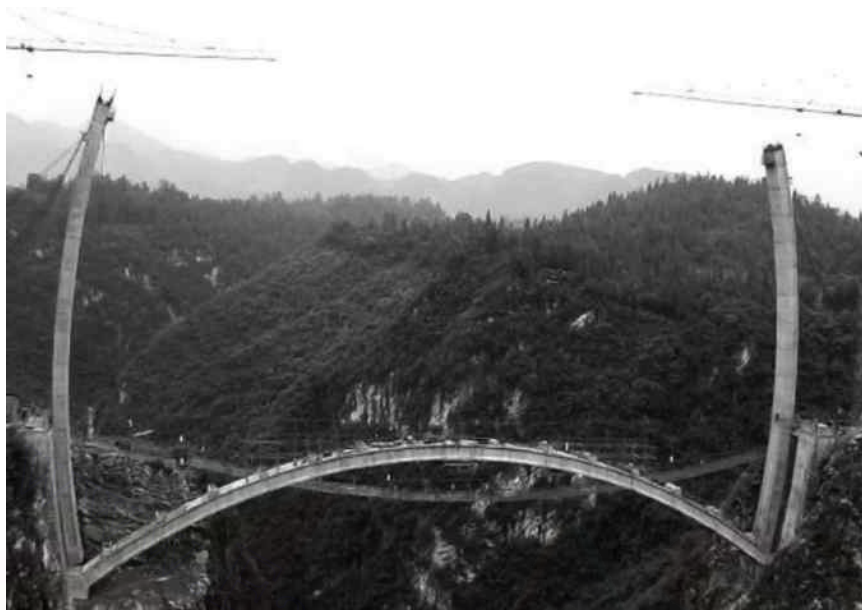
Figure 9.6 Vertical casting and rotating of arch bridge. (Zhenzhu Bridge, China, 2008, Courtesy of Guizhou Bridge Construction Group Ltd.)
