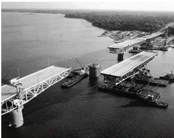
Figure 10.3 Construction of George P. Coleman Bridge in segment. (Courtesy of VDOT, Virginia.)
