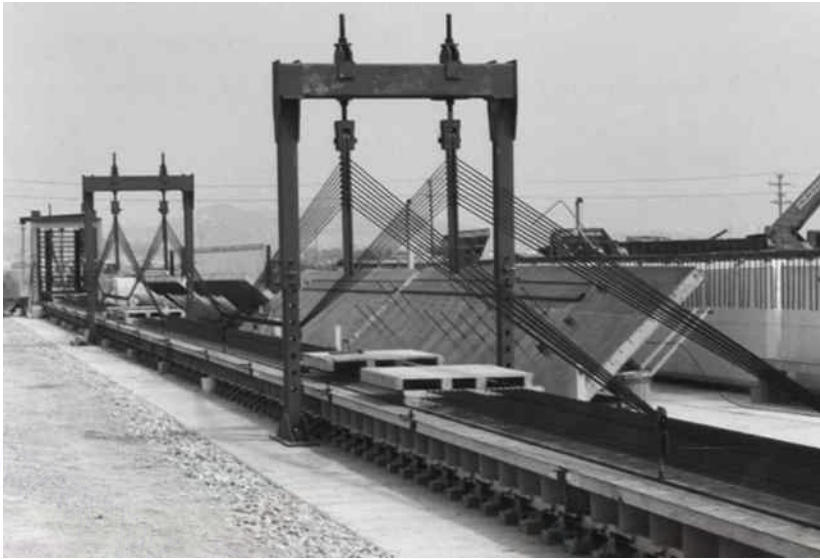
Figure 5.3 Harped prestressing strands. (Data from FLDOT/Corven Engineering, Inc., New Directions for Florida Post-Tensioned Bridges , Volume I: Post-Tensioning in Florida Bridges, Florida Department of Transportation, Tallahassee, FL, February 2002.)
